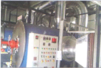
Hot Air Generator
