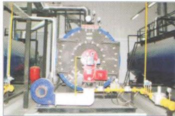
Hot Water Boiler
